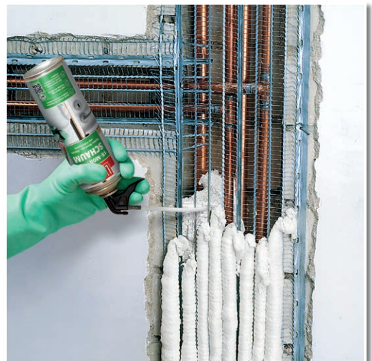
Thermal insulation of heating pipes.
